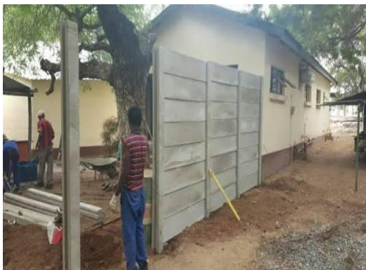
Pre-cast compound wall
