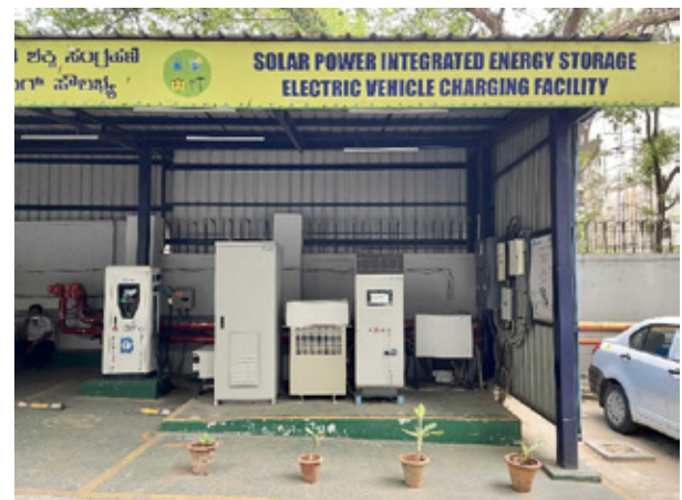
Figure 7.11: The installed prototype 193
