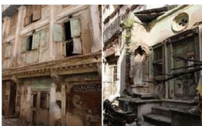
Dilapidated Heritage buildings, Surat
